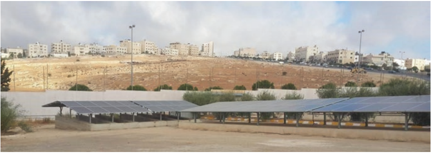
Fig. 52.5 PV panels were misplaced next to student's plaza at Applied Science Private University; it was highly rejected by people (source: researcher)
