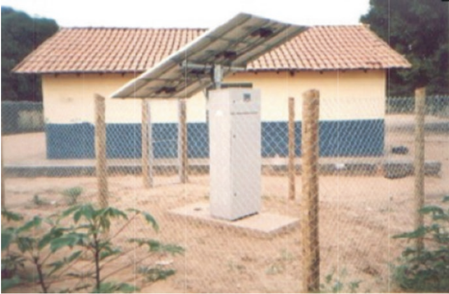
Fig. 4.2 School PV system, typical of the distributed installations for the modules from this study
