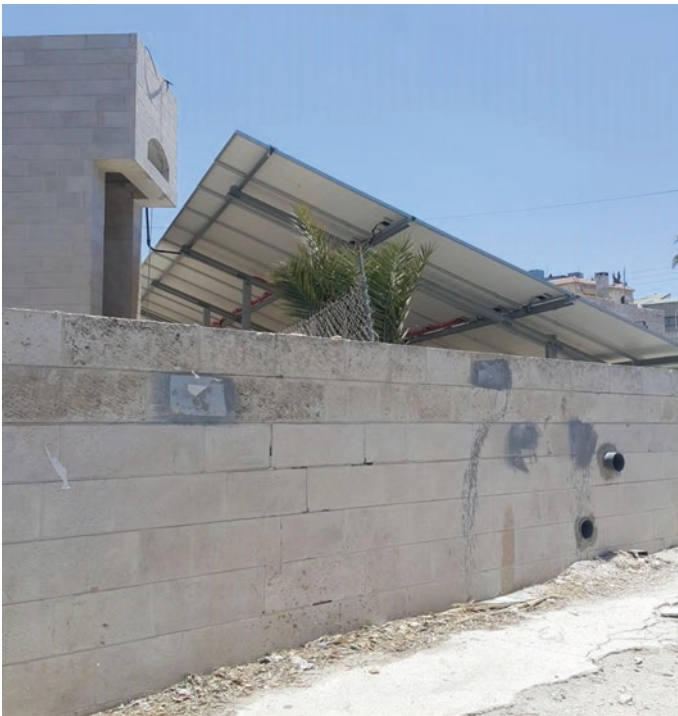
Fig. 52.10 PV panels are misplaced; this treatment was highly rejected by people since it distorts the view and ruined the elevation (source: research)
