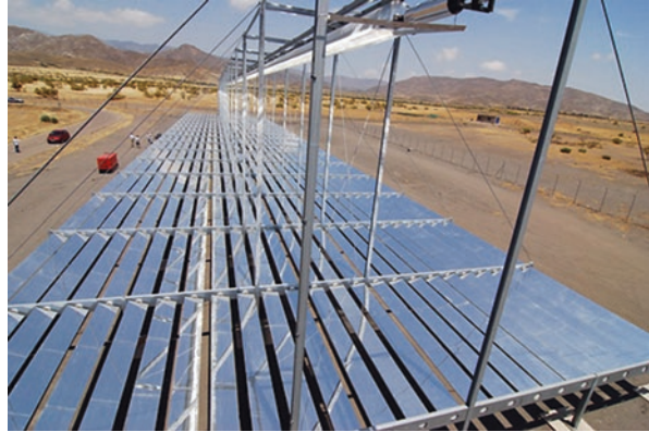
Fig. 26.1 View of the liner Fresnel reflector (LFR) plant in Plataforma Solar de Almería(PSA), Spain
