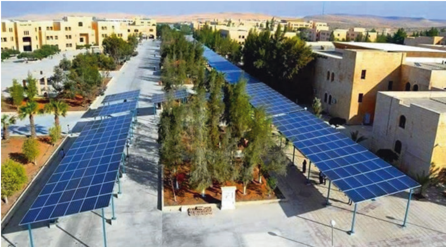
Fig. 52.3 A good example of the photovoltaic panels placed on the roof of a passage at the Hashemite University. It was highly accepted by people (source: albosala.com )
