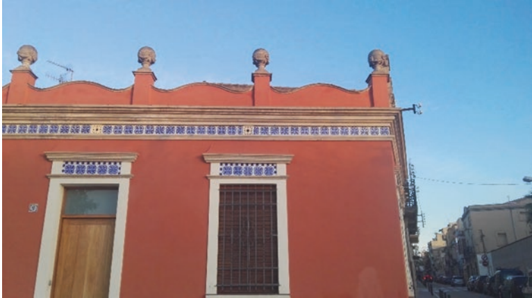
Fig. 16.14 Ventilated roofs in urban environments. The small holes under the cornice are used for ventilation
