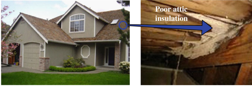
Fig. 12.21 In houses, heat is conducted from the inside to the outside more rapidly where insulation is poor. Thus, houses should be well insulated especially in the attic to minimize heat loss
